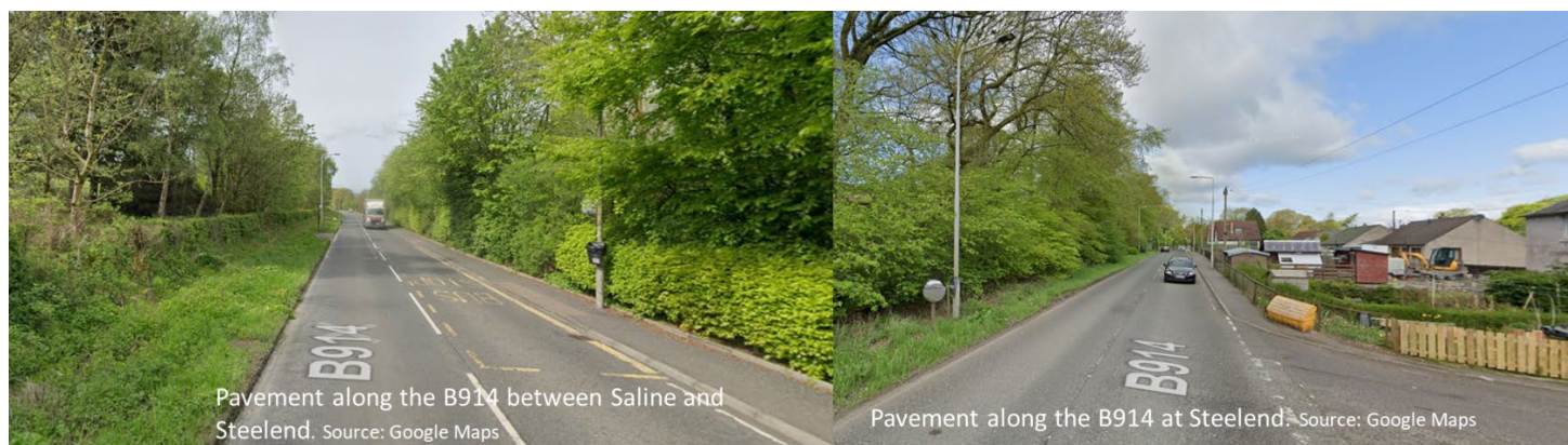
Figure A1-6: Photos showing the pavement condition along the B914.
