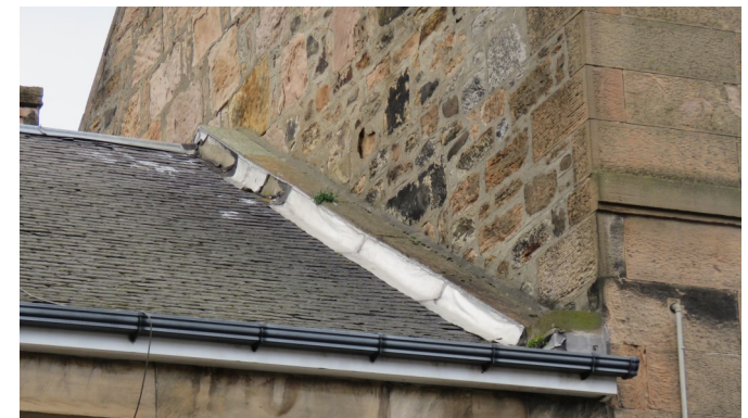
Poorly detailed roof maintenance – would not meet current standards of good conservation practice
