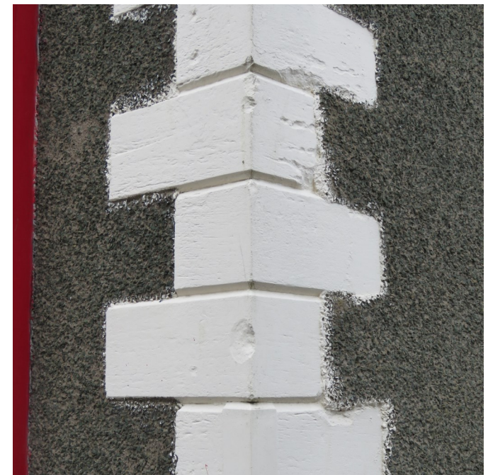
Unsympathetic use of cement harling around historic masonry quoins (corner stones) – would not meet current standards of good conservation practice
