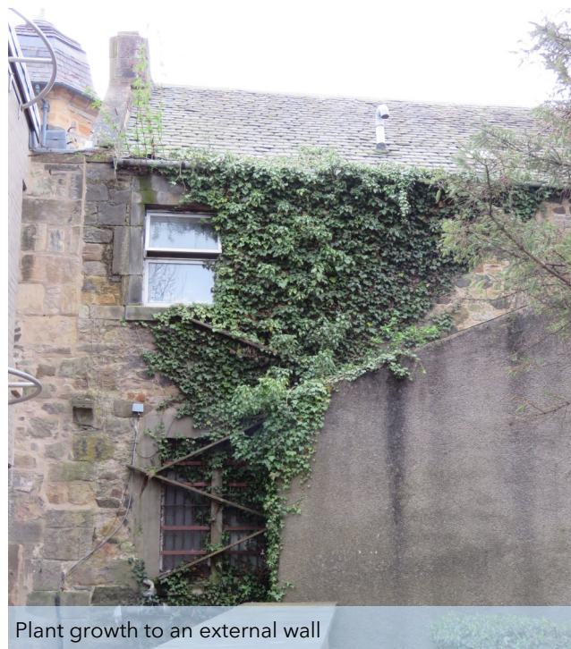
Roof-level maintenance issues
