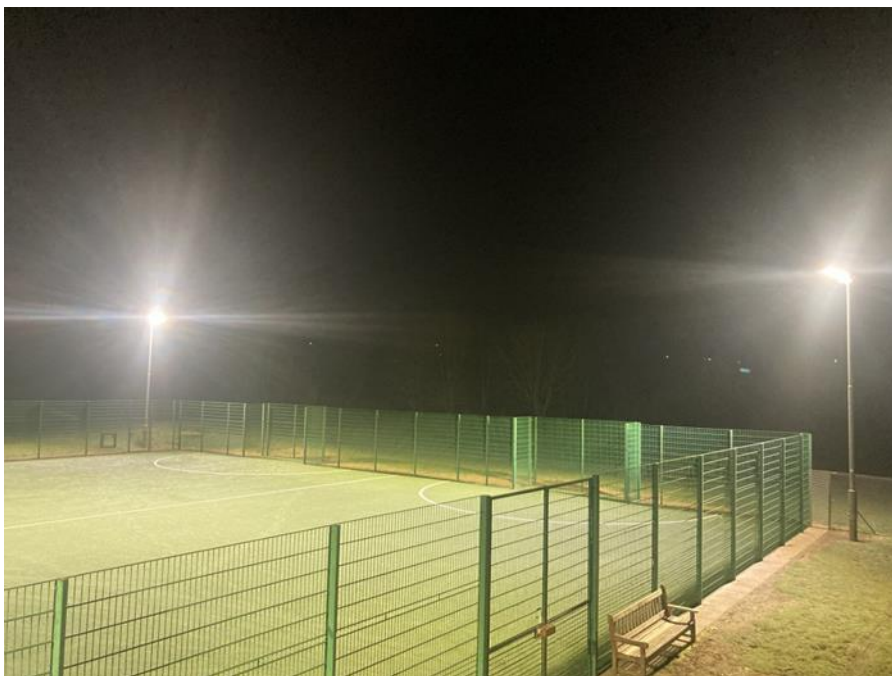
Figure 4 - Valleyfield Sports Hub Eco Floodlights
