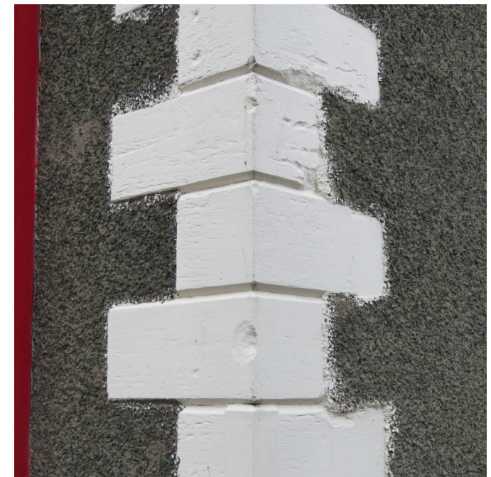
Unsympathetic use of cement harling around historic masonry quoins (corner stones) – would not meet current standards of good conservation practice
