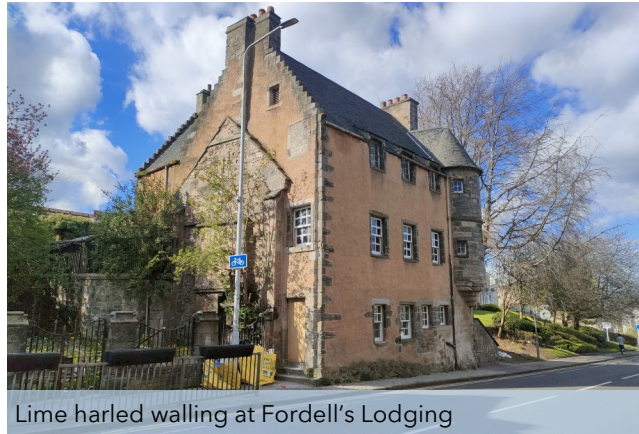
Gable with decayed mortar
