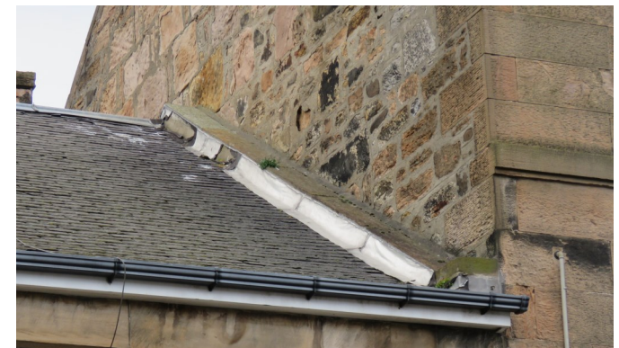
Poorly detailed roof maintenance – would not meet current standards of good conservation practice
