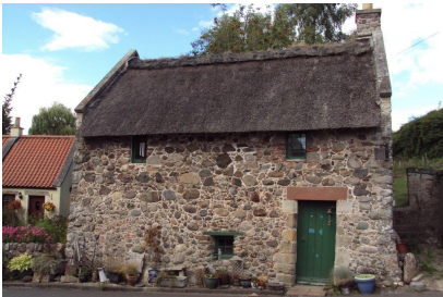
The above (and right) former washhouse has had the gables pitch reinstated and a thatched roof added.
